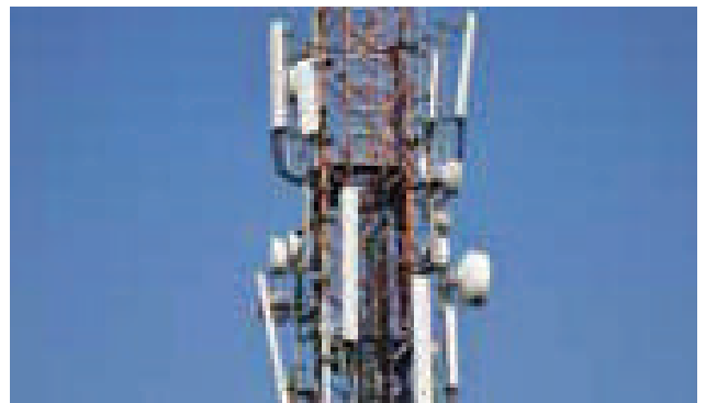
Mobile Tower Switching Areas
