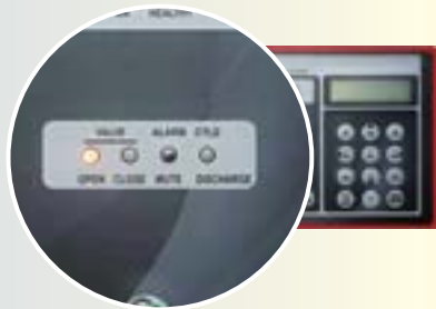
Electronically monitored through the control panel.
