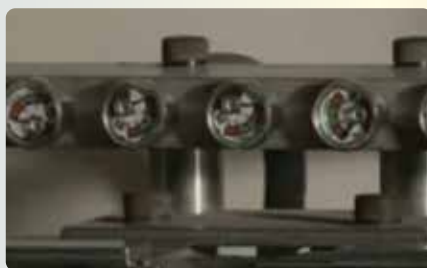
✓ Pressure Gauge Test
